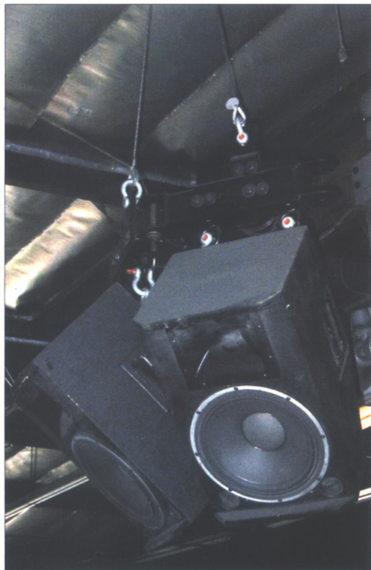
Loudspeaker cluster suspended from a wood beam using offset swivel ring fasteners on both sides.
